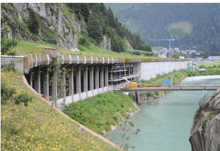
Fig. 4. Avalanche protection gallery as seen from the roof of the northern railway gallery founded on rock near natural and artificial weir above the Schöllenen gorge.
