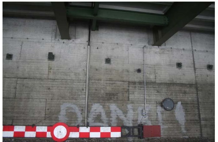
Fig. 6. Retaining wall with open joint due to differential settlement and heads of tiebacks placed.
