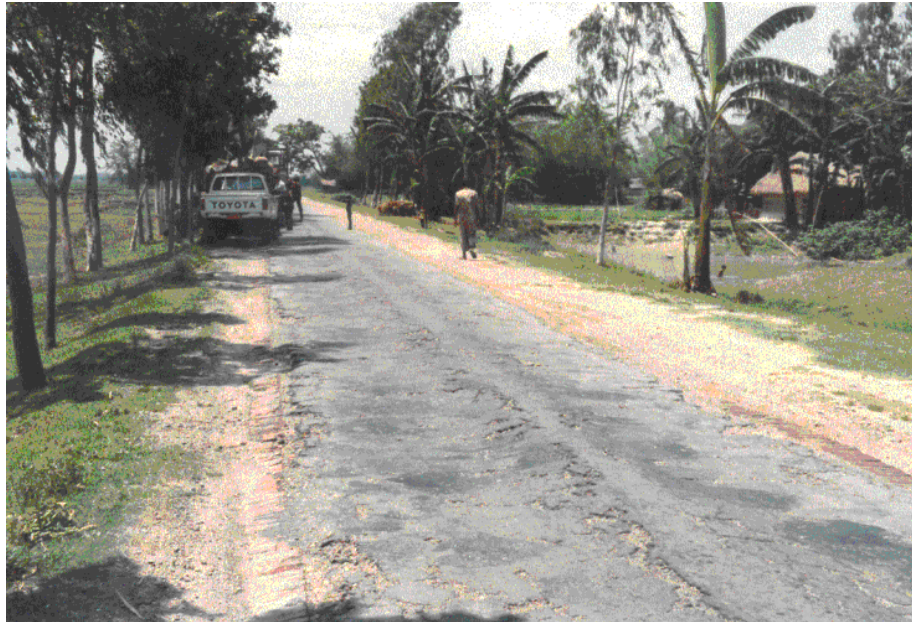
Fig. 1 – Old road. At center the damaged pavement. Laterally the two unpaved shoulders.
